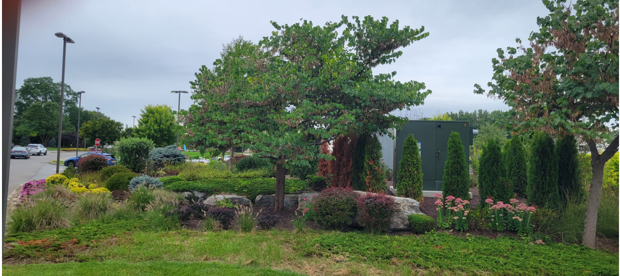
Walmart Plaza charging station transformer and landscaping, photo by submitted by Aaron Sweeney, September 21, 2022.
